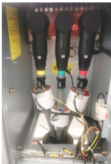
Ring main unit – after installing the temperature-sensing insulating plug and back cover
