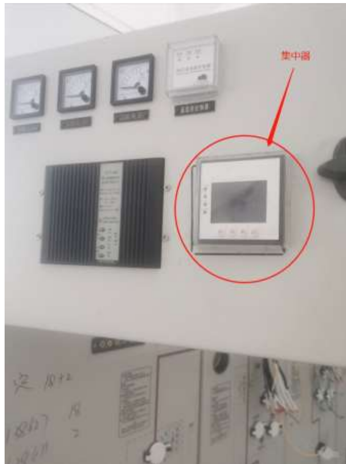
The front of the installed Passive Wireless Online Temperature Monitoring System
